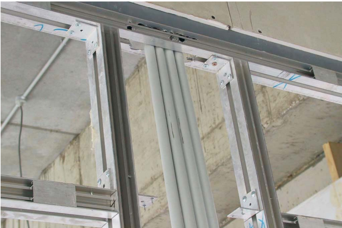
Upper Electrical integration
