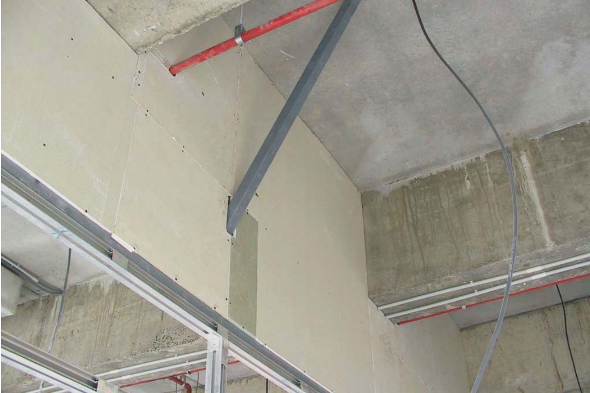
Acoustic barrier above false ceiling
