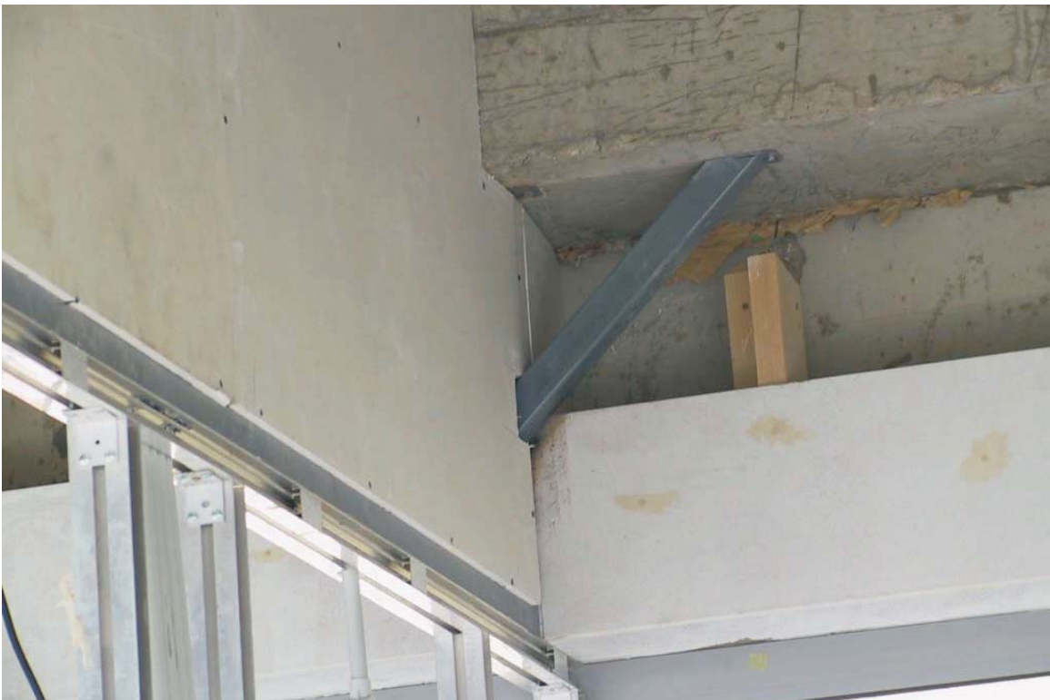
Alum Structure on Accoustic barrier
